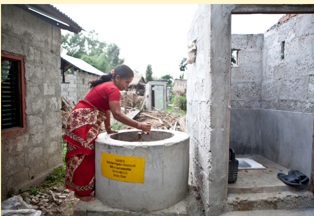
A beneficiary in Kumroj demonstrates how the mixture is churned in the biogas pit, typically constructed next to a toilet.
