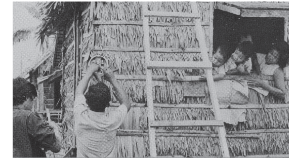
Linemen installing an electric meter for cooperative members as part of USAID's rural electrification programming during the 1960s and 1970s.
