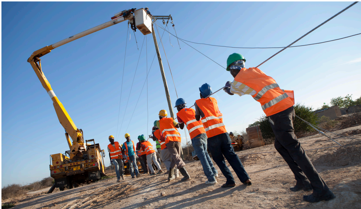
A utility crew from Pike Electric, an American contractor, works to string power lines in rural Dodoma Region, Tanzania. The initiative is part of the Millennium Challenge Corporation's (MCC) Energy Sector Project. (Photo: Jake Lyell for MCC)
